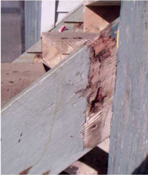
Another example of the rotten wood
