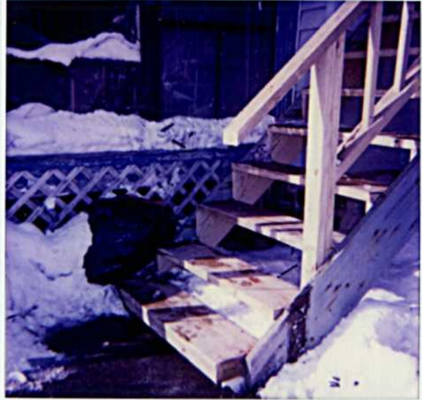
Shows how the stairway used the old, rotten wood as its basis. Also shows the span in between the spindles.
