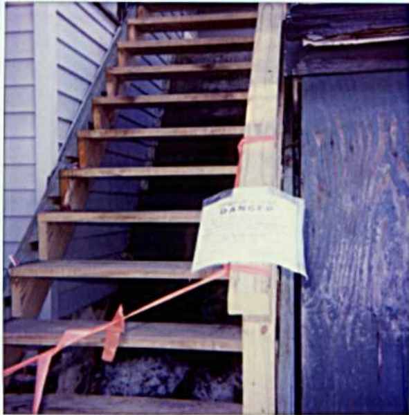
Shows that the stairway was condemned
