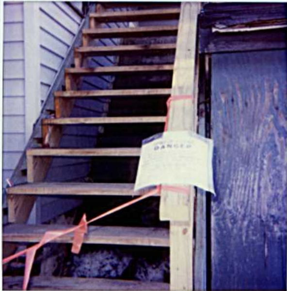
Shows that the stairway was condemned
