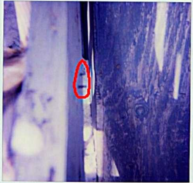
Shows more screw points protruding out where they could injure someone.
